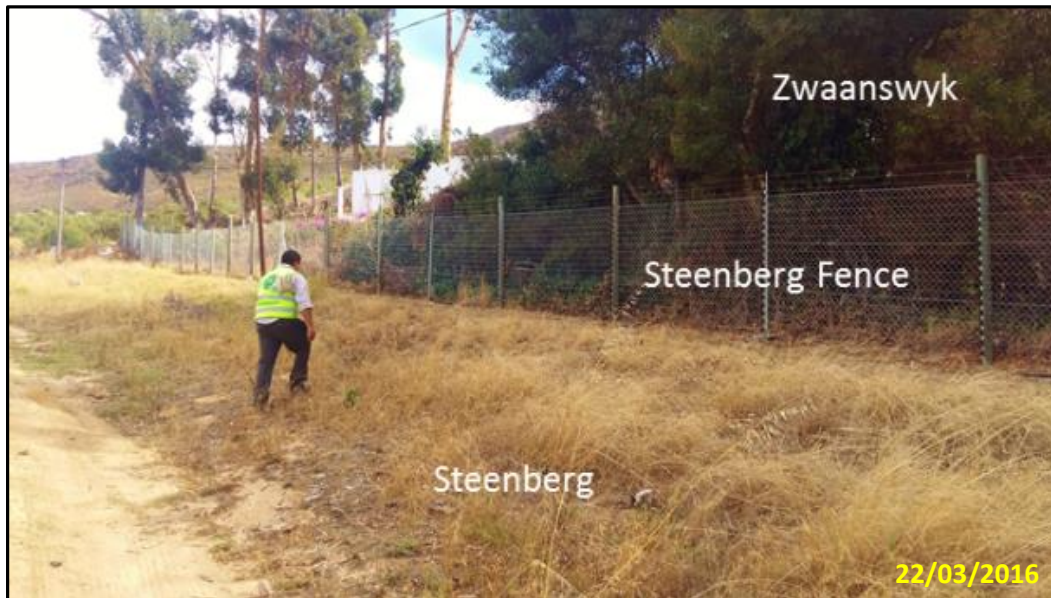
Figure 17: HWS Manager, Devin Heuwel, inspecting the Steenberg Fence. The poor design of the fence allows baboons to jump onto the fence poles from the Steenberg side, and then into Zwaanswyk.
